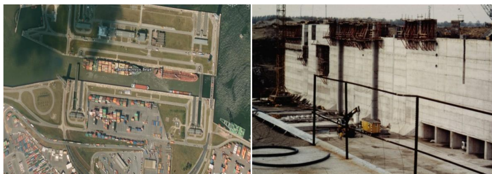
Fig. 1. Overview of the Berendrechtlock (left) and the embankment wall during construction containing 200,000 tons of recycled aggregate (right)
