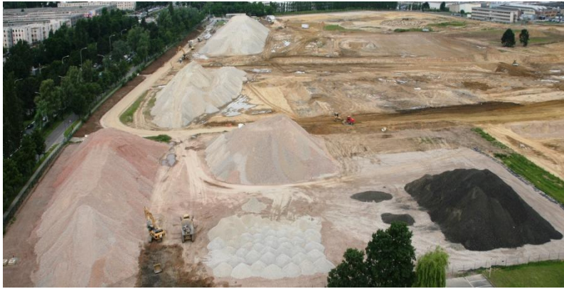
Fig. 4. Overview of the Demolition & Recycling Site showing the different products made on-site © NATO
