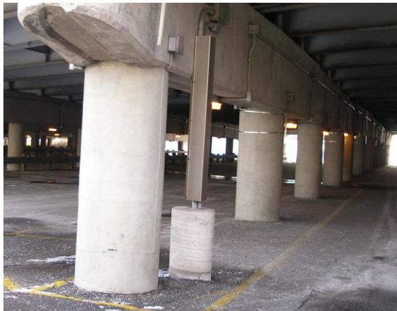
Fig. 9. Repaired Columns after Thirteen Years of Service
