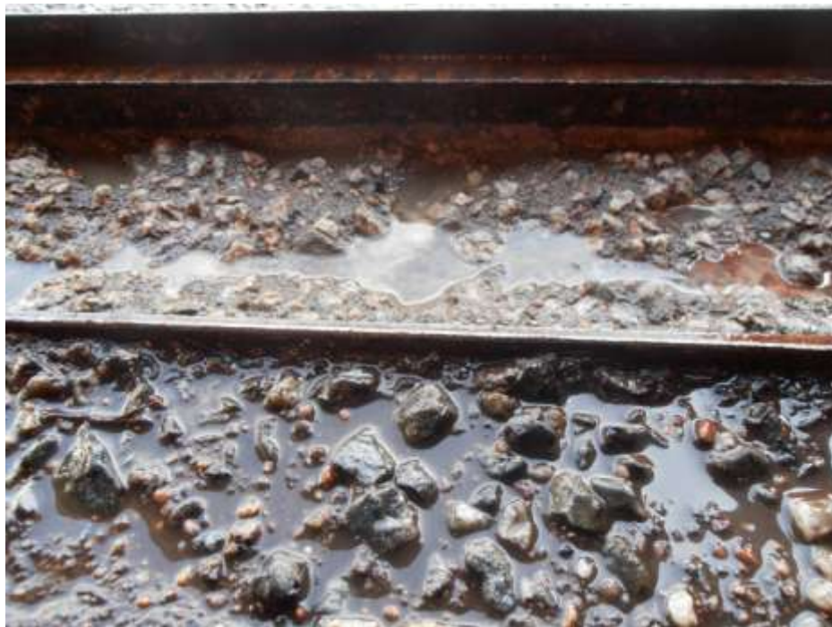
Figure 1. Damaged floor in reception hall for food waste (photo: Mattias Persson, Atleverken)
