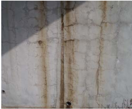
Figure 12 Cracks occurred on the patch repair in Structure F
