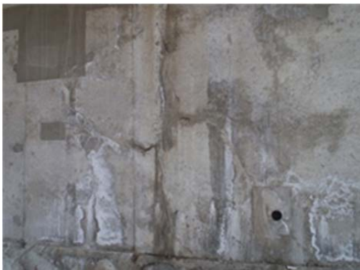
Figure 18 Cracks occurred on the patch repair Structure H
