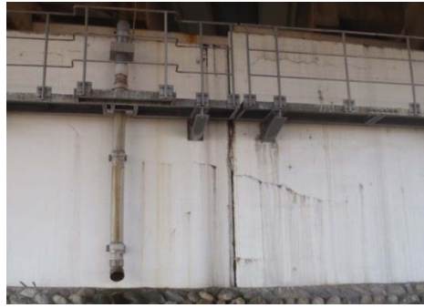
Figure 8 Cracks occurred on the repaired in Structure C
