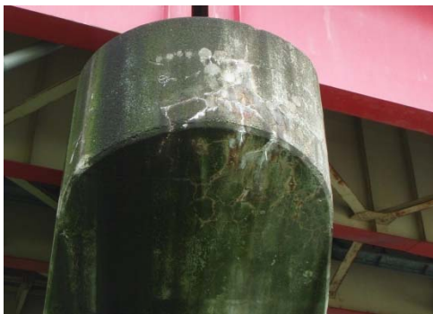
Figure 9 Deterioration due to ASR in Structure E
