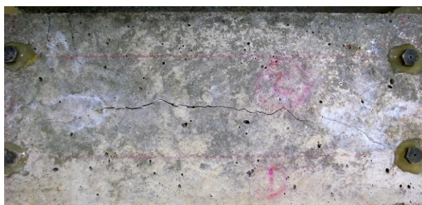
Figure 4. Concrete cracking observed in RC1 specimen stored in 30°C
