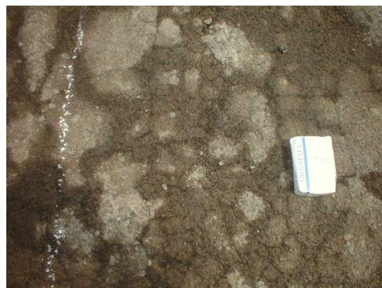
(b) Cracks of concrete slab under the damaged asphalt pavement
