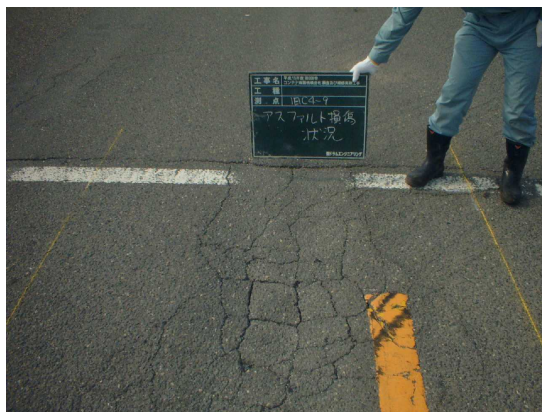
(a) Damage (cracks) of asphalt pavement
