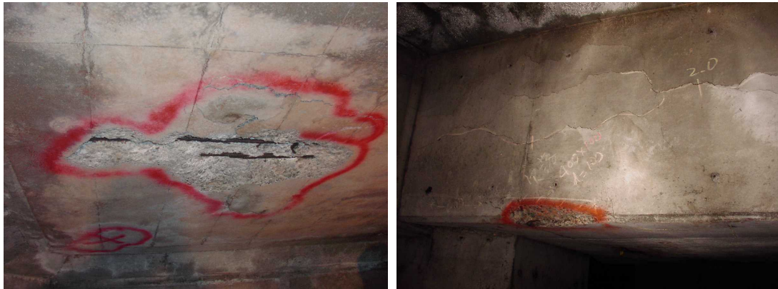
(a) Chloride induced corrosion of reinforcing bar of a slab
