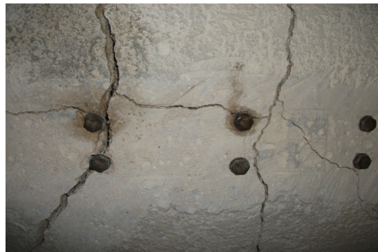
Figure 4. Concrete cracks formed around the bolts.
