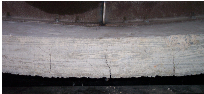
Figure 3. A view of the symmetrical cracks on the beams.
