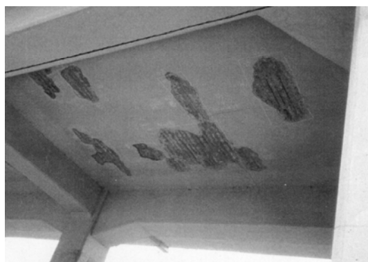
Photo 1. Deterioration of the slab
