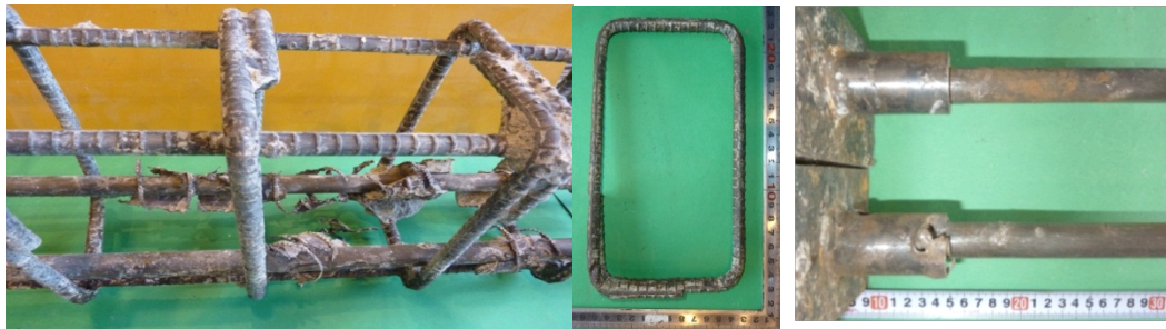
Photo 2. The state of reinforced bars of PC-O beam
