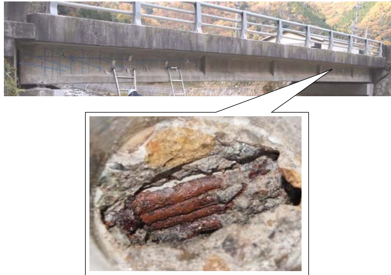
Photo 1. Example of corroded tendons in a real PC bridge
