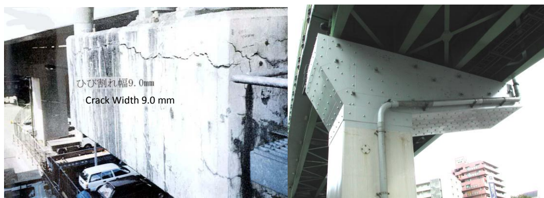
Figure 3. Typical Damage caused by Alkali Silica Reaction
