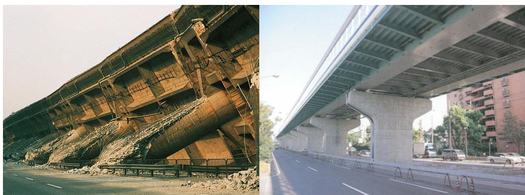
Figure 4. Viaducts Seriously Collapsed and After the Restoration
