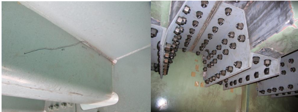
Figure 1. Fatigue Damage on Orthotropic Deck
