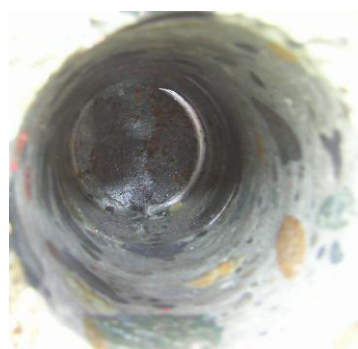
Figure 10. Steel pile of Type A after 21 years
