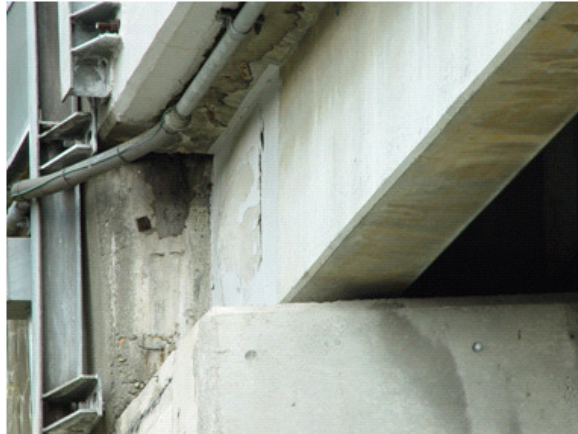
Photo 3. Deformation state of crossbeam transverse prestressing anchorage constructed by FRP bonding method
