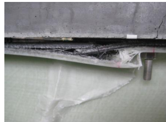
(b) HFRP flange delamination failure
