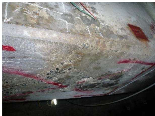
Figure 7. Bottom surface of beam near No.1
