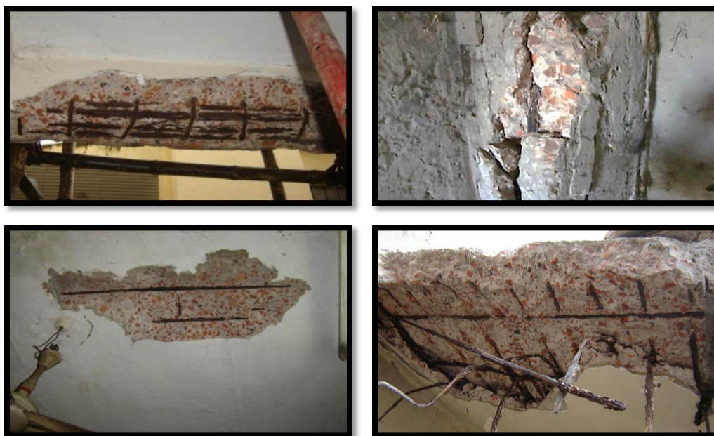
Figure 2. Corrosion of steel due to carbonation: structures in Dhaka city
