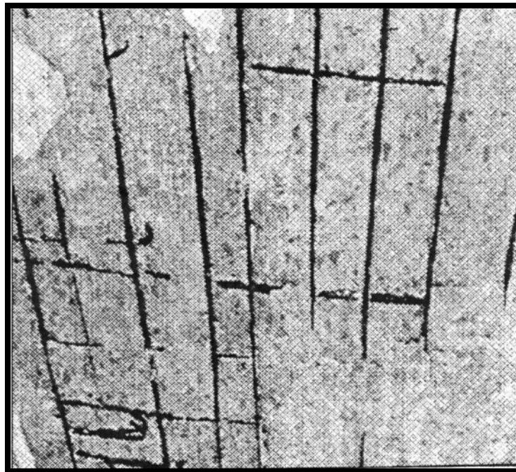
Figure 11. Spalling of cover concrete from slab (The Daily Ittefaq, 16 th April, 2007)
