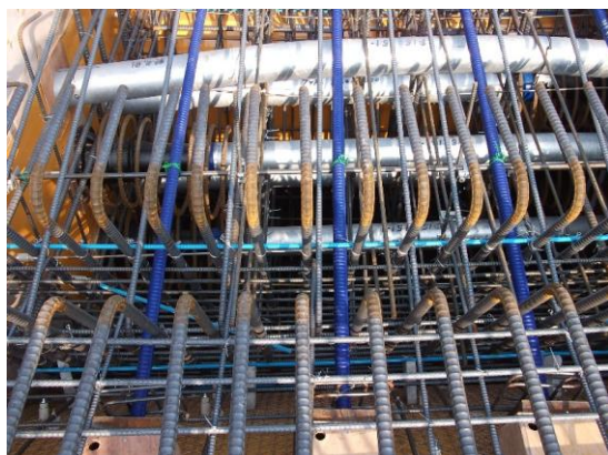
Photo 1. An example of congested reinforcing bars
