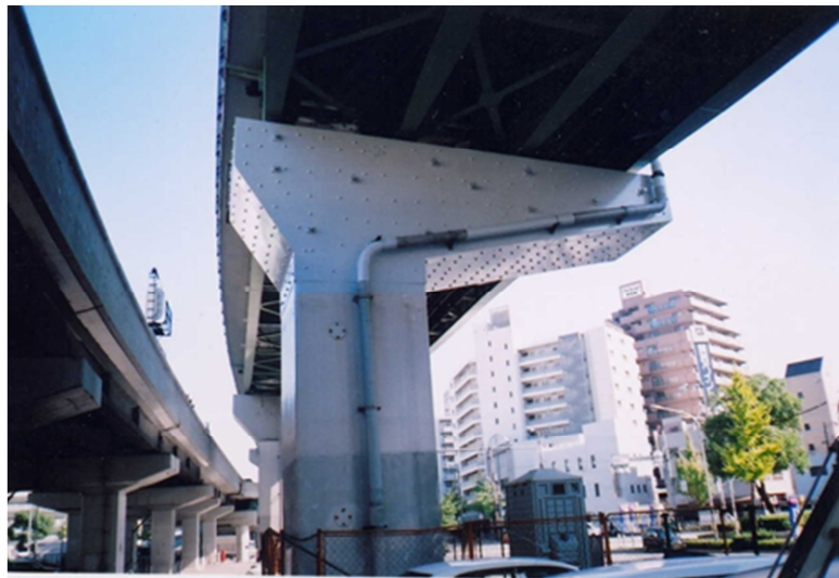
Photo 2. Reinforcement of a RC beam damaged by ASR
