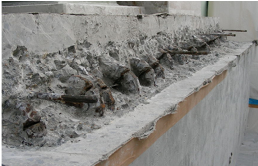
Photo 1. Ruptures of reinforcing bars
