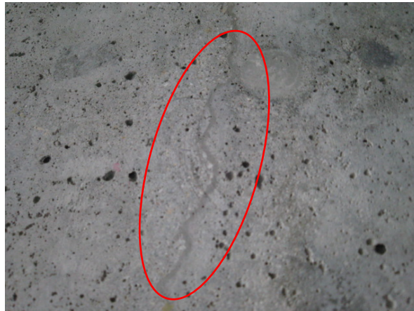
Figure 6 Condition of injected crack trace
