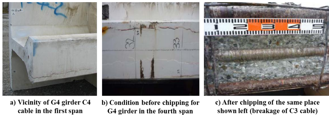
Figure 14. Damage condition at the part with filled grout (C bridge)
