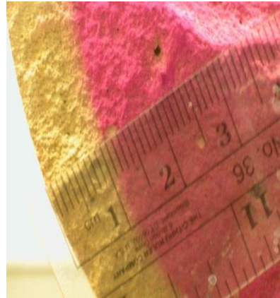
Figure 2. Measurement of Carbonation (in cm)
