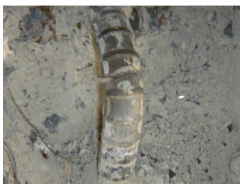
Figure 1. Rupture of reinforcing in a concrete structure
