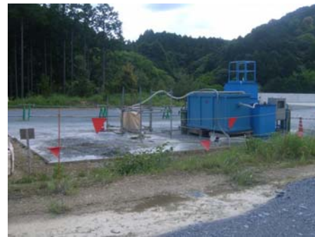
Photo 10. Water treatment unit
