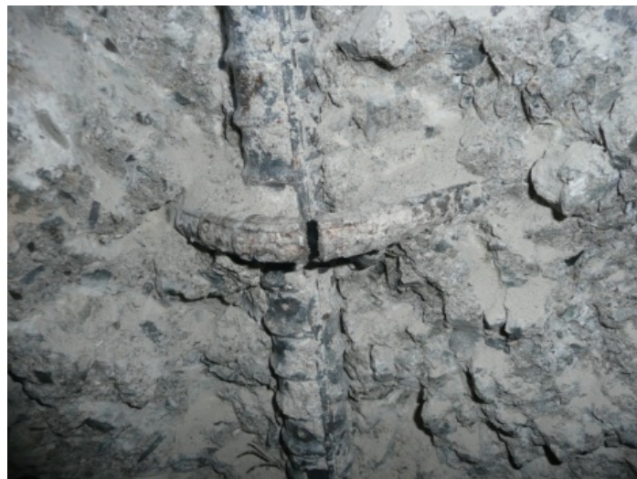
Figure 4. The reinforcing steel (tie hoop) rupture
