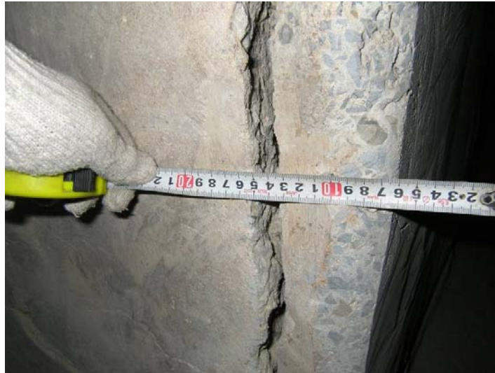
Figure 3. More than 15 mm crack at the corner of the column bottom
