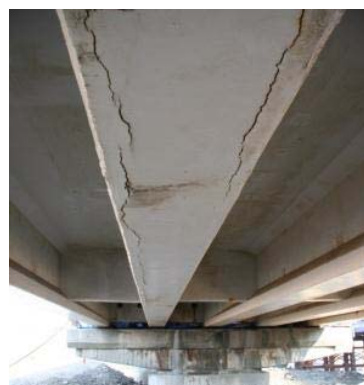
(b) Bridge G (2 years after last repair)
