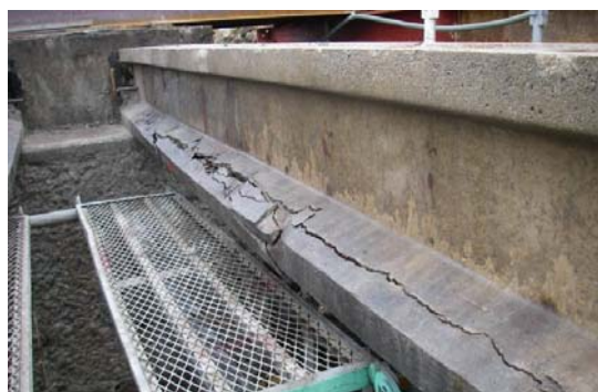
Figure 1. PC bridge beam affected by salt attack in Niigata Pref., Japan (constructed in 1975)
