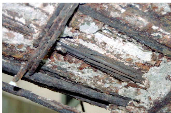
Figure 1: Heavily corroded tendons with broken wires
