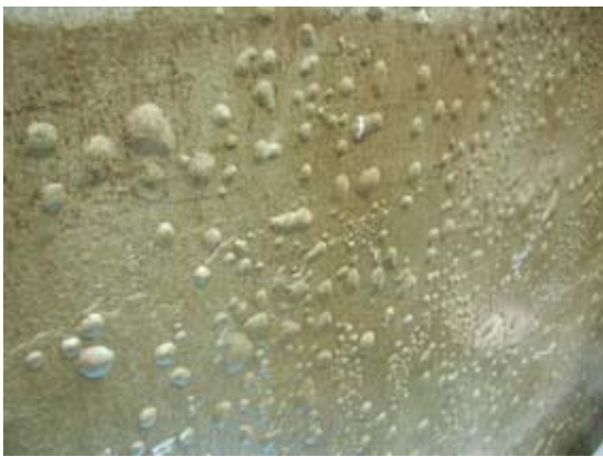
Photo 2. ‘Swell’ of concrete protection coatings
