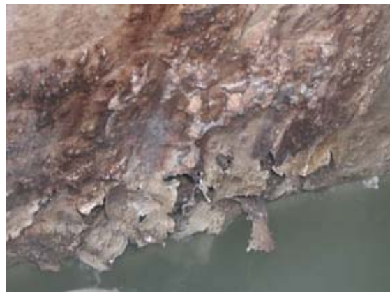
Photo 3. ‘Peeling off’ of concrete protection coatings
