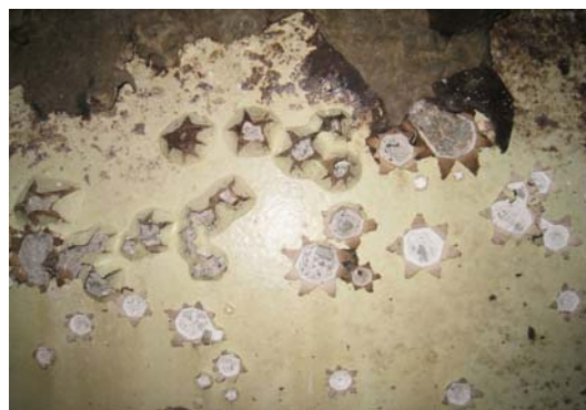
Photo 1. Pinholes of concrete protection coatings
