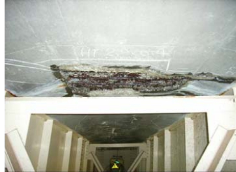
Figure 2. Delamination at the construction joint of slab
