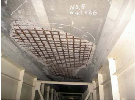
Figure 1. Delamination around middle of slab
