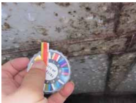
Photograph 9. Corrosion-resistant surface pH
