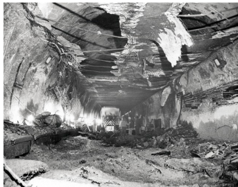
Figure 1. Damage of lining tunnel structure due to fire in Holland, New York State, US, 1949 (Google).
