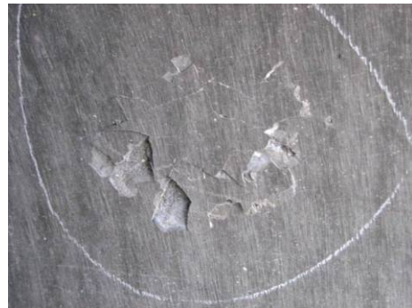
Figure 17. Verified delaminations of mortar lining (inside pipe)
