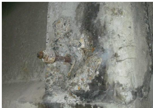
Figure 1. Protrusion of PC steel bars from an anchorage area
