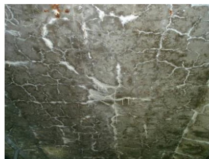
Photo 8. Fatigue of RC floor Slab
