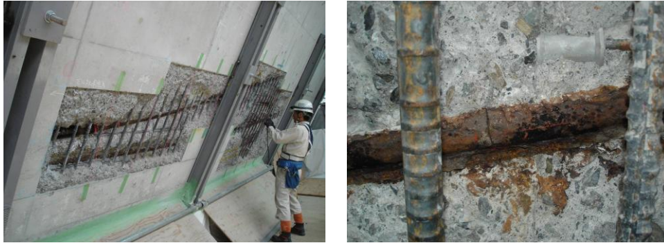
Photo 9. Poor Grouting and broken PC bar of PC Bridge (Initial Defect)
