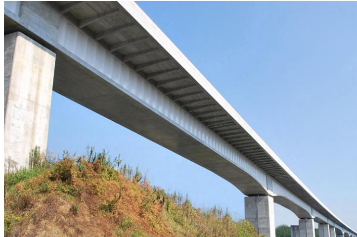
Photo 4. Using corrugated steel web bridge (AKABUCHIKAWA bridge in the new TOMEI exp.)
