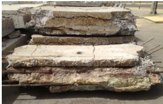
Figure 2. Delamination in roof slab after removal from the sulfur pit during repair
