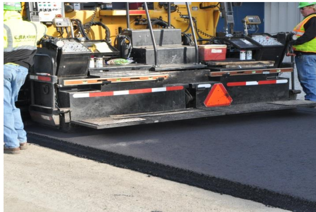
Figure 1. Paving at the Oak Creek Power Plant in Wisconsin with both ASHphalt for comparison to a control section of asphalt concrete
