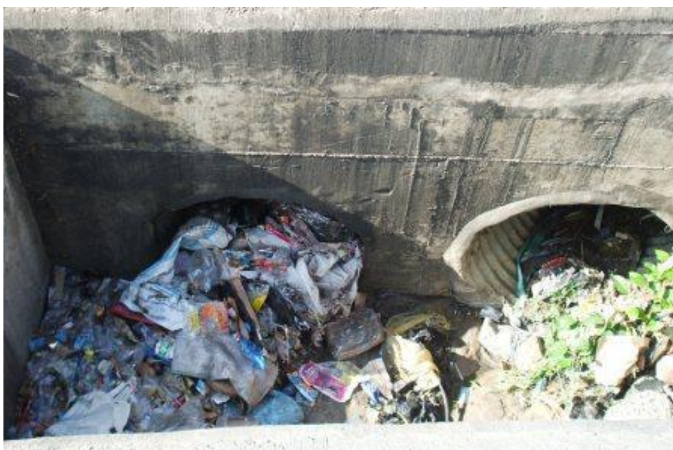
Fig. 5. Waste plastics in Maiduguri, Nigeria blocking drainage infrastructure.
