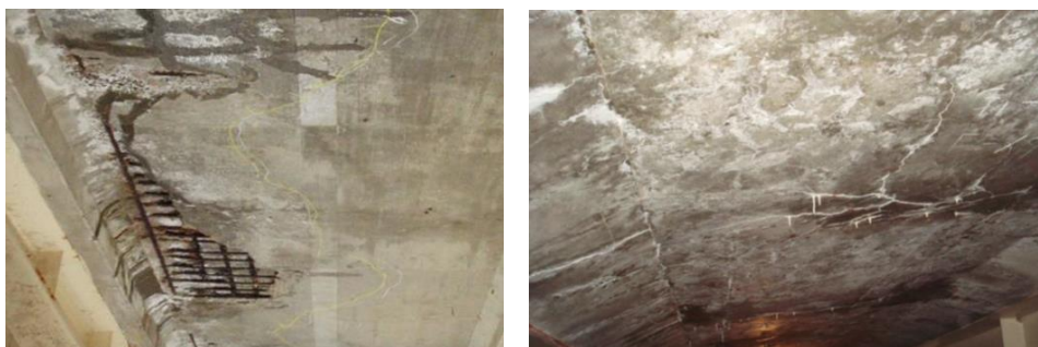
Figure 1. Corrosion of Rebar and Spalling of Concrete on the Upper Surface of Slab
