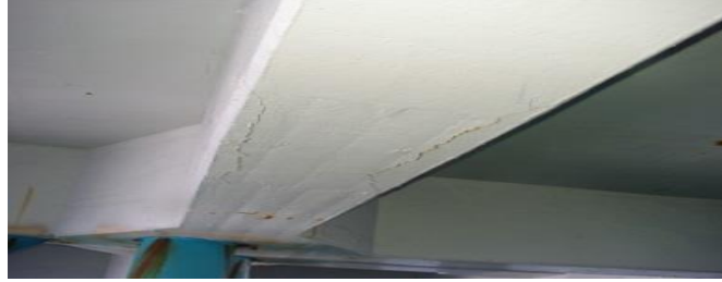
Figure 2. Cracks of a beam
