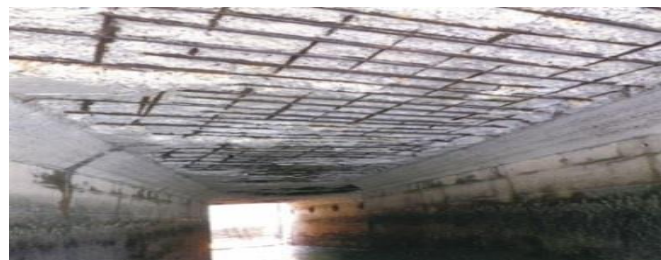
Figure 3. Delamination of a slab
