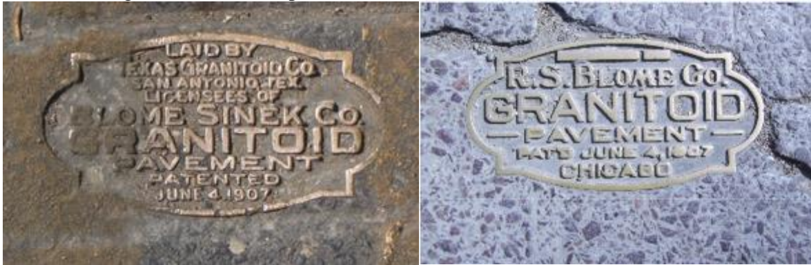
Figure 1. Embedded bronze plates in pavements constructed in San Antonio, TX (Taubert and Prusinski, 2014), and in the village of Calumet, MI (Mailloux et al., 2008).
