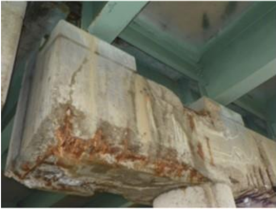
Spalling and exposed rebar on east cap, pier #2
