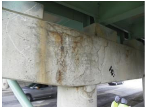
Cracking and delamination on pier #2
