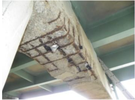
Spalling and exposed rebar on bottom of a cap, pier #2
