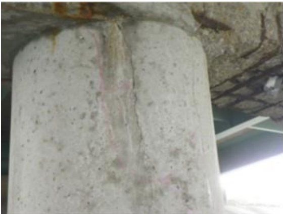
Cracking on column #1, pier #2
