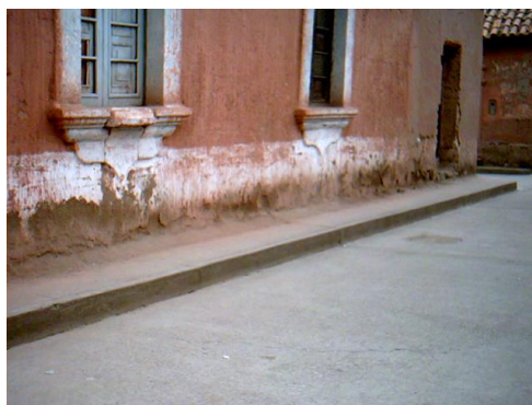
Figure 1: Unprotected earthen wall in Lampa (Peru) damaged by water flow. Credit: A. Bourgès
