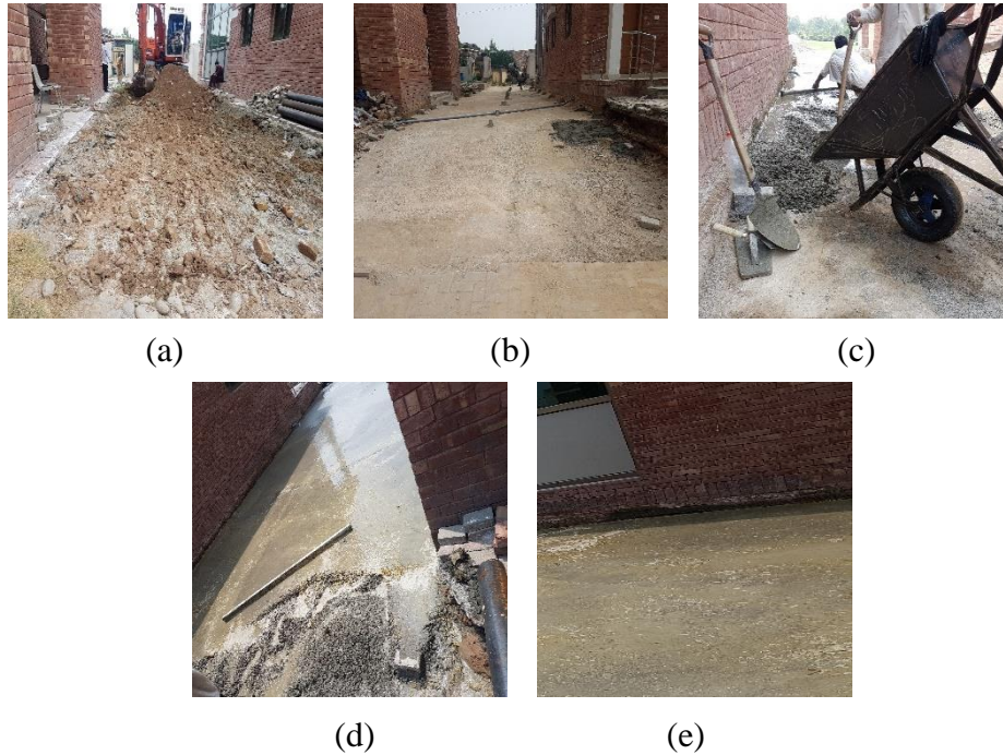
Figure 3. Laying Process (a) Soil layer preparation (b) Surface preparation with levels (c) Laying of concrete (d) Levelling (e) Finish surface
