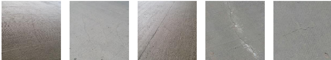
Figure 1. Early age cracks in newly constructed rigid pavements
