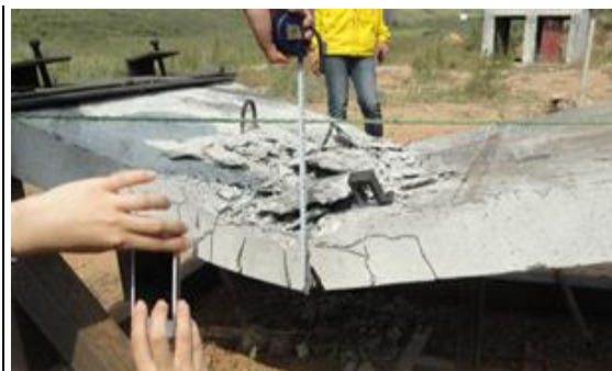
Figure 5. Shattered NC slab panel with shrapnel
