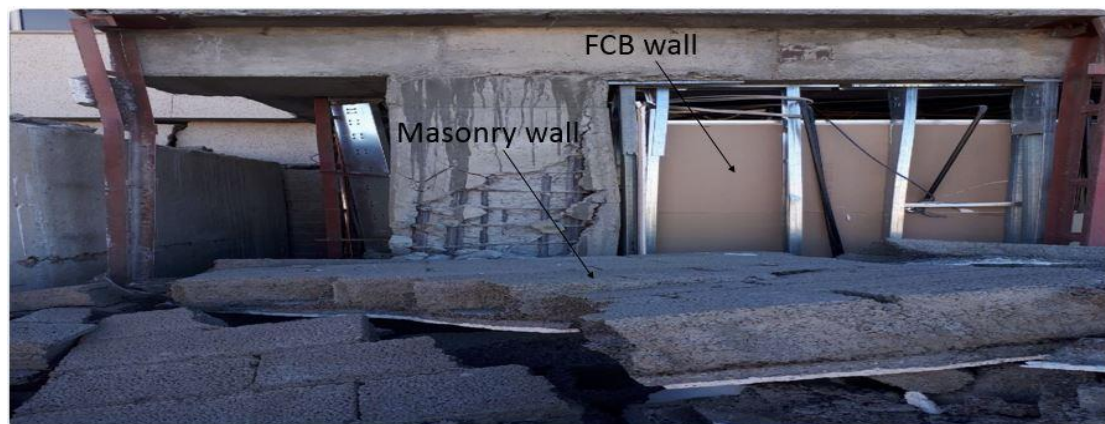
Fig. 1 Performance of masonry and FCB walls in recent Sarpol-e Zahab earthquake
