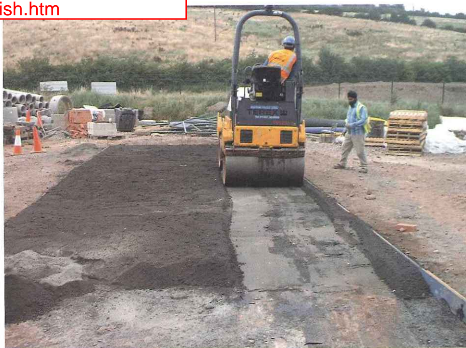
Figure 1: CEM 0 trial with a concrete without aggregate. This semi-dry paste was laid in a 100mm layer.
