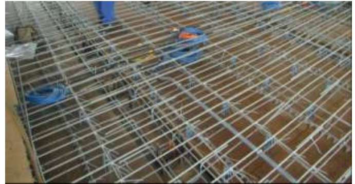
Figure 5. Haunch reinforcement to compensate for inadequate length of shear studs.
