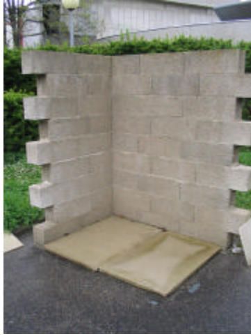
Figure 3. Concrete blocks and screeds after 4 years of natural weathering.
